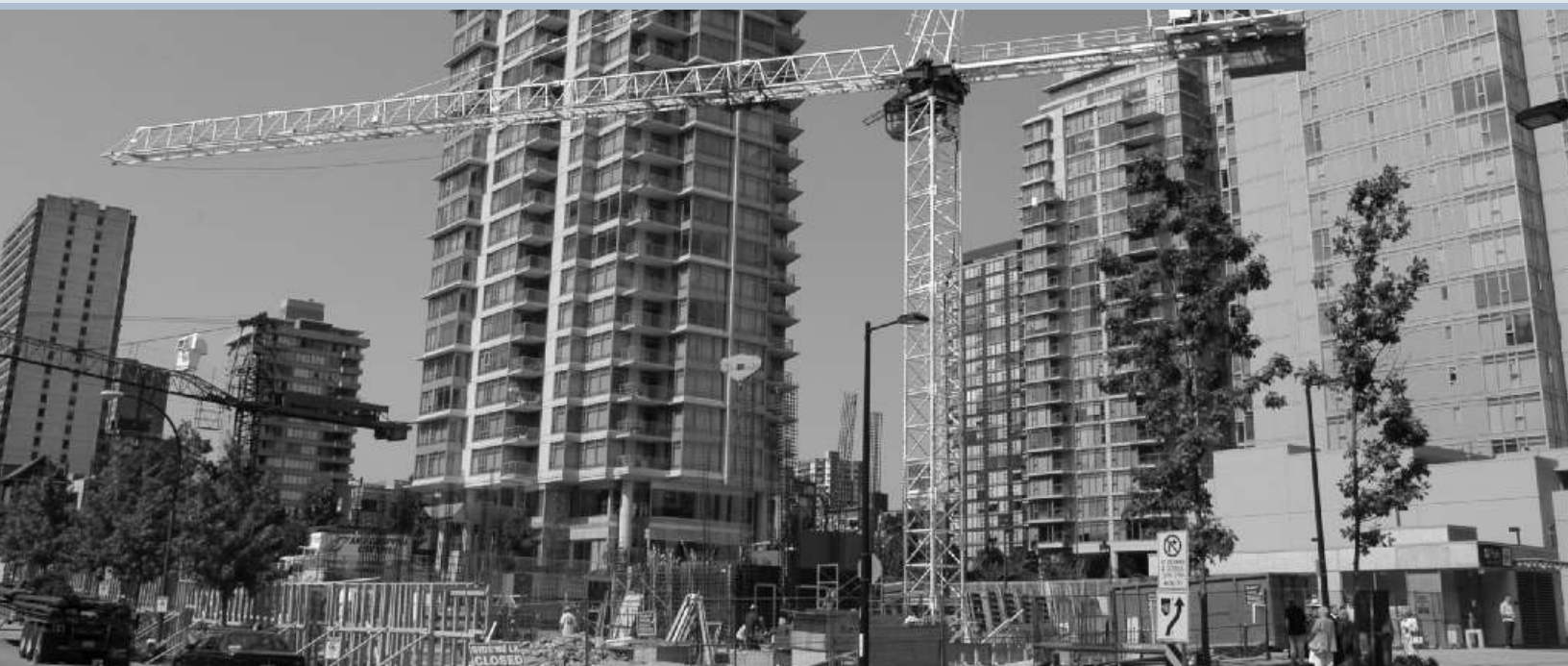
Construction site of Vancouver's Performing Arts Lodge — 111 units for seniors in the performing arts developed in partnership with BC Housing, CMHC, City of Vancouver and other donors.
